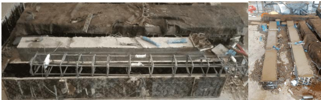
Fig. 7: (a) Steel cages and internal strain gauges fixing; (b) beams Casted and covered for curing
